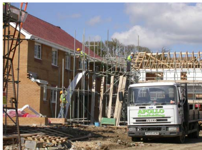
Residential development on green field sites on the outskirts of Newport, Isle of Wight
