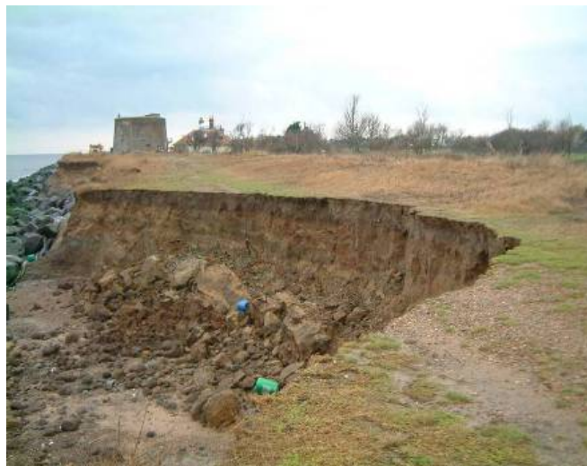
Figure 1.2 Erosion of Environment Agency flood defence embankment, November 2004 (source: Terry Oakes Associates Limited)
